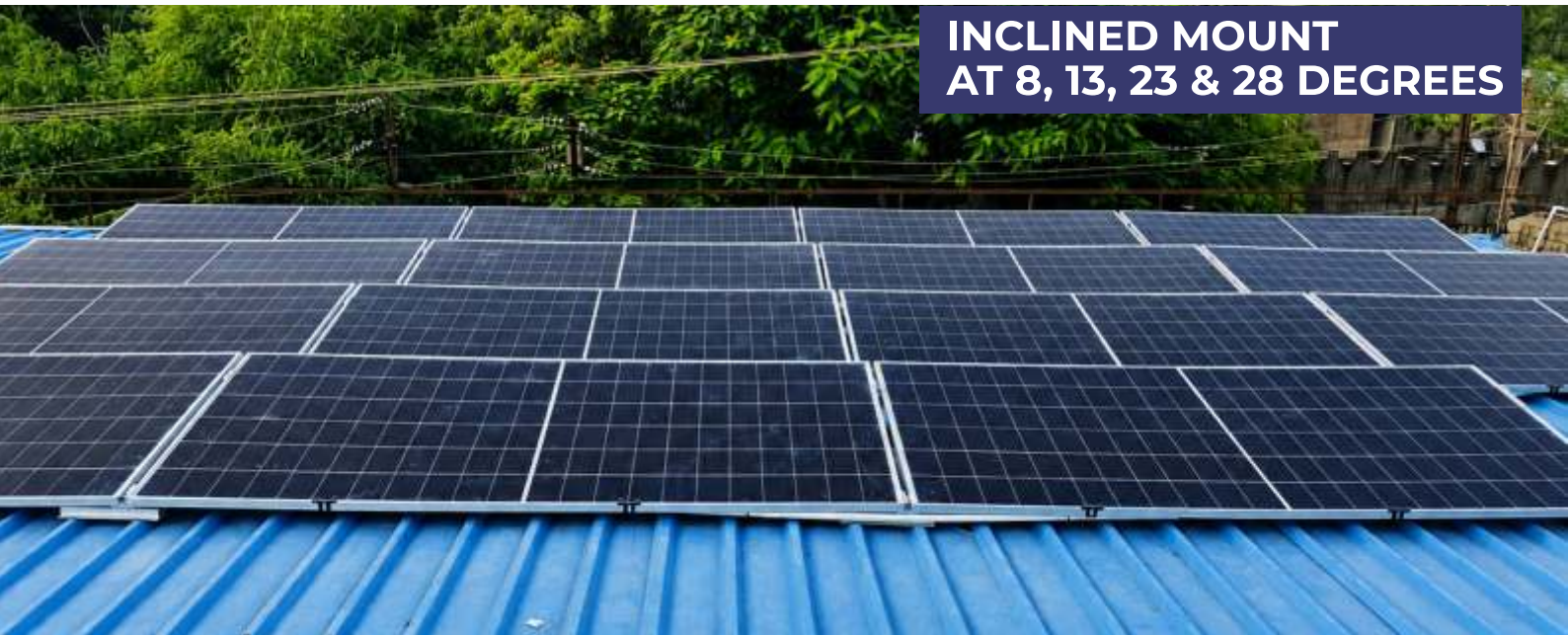
North Inclined Solar Mounting structure
